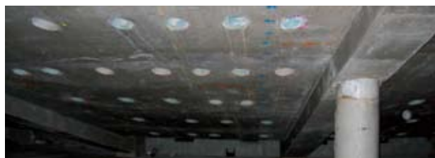
Under floor air supply holes
