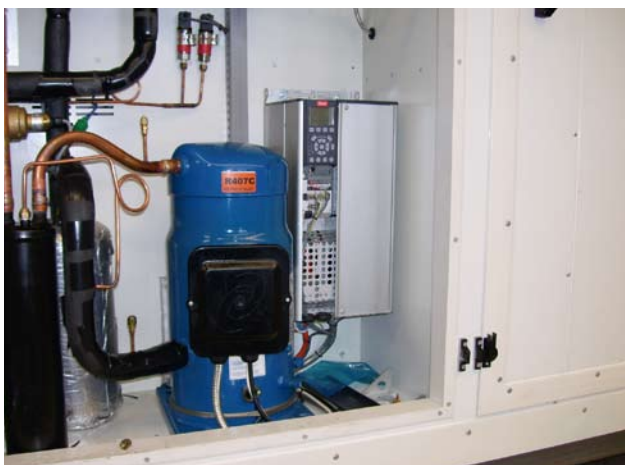
Compressor and Compressor VSD (Variable speed drive)
