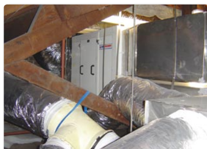
The stainless steel, fully lined metal and flexible duct work
