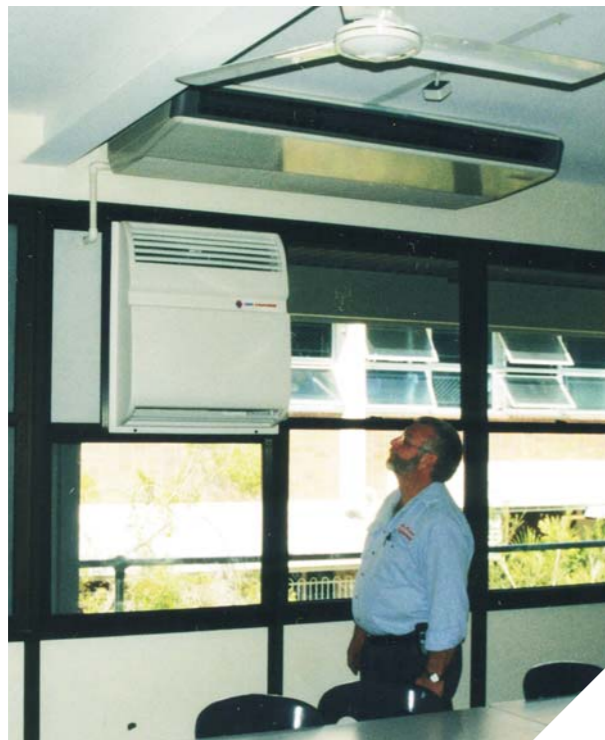
An Air Change ERV with ceiling air conditioner
